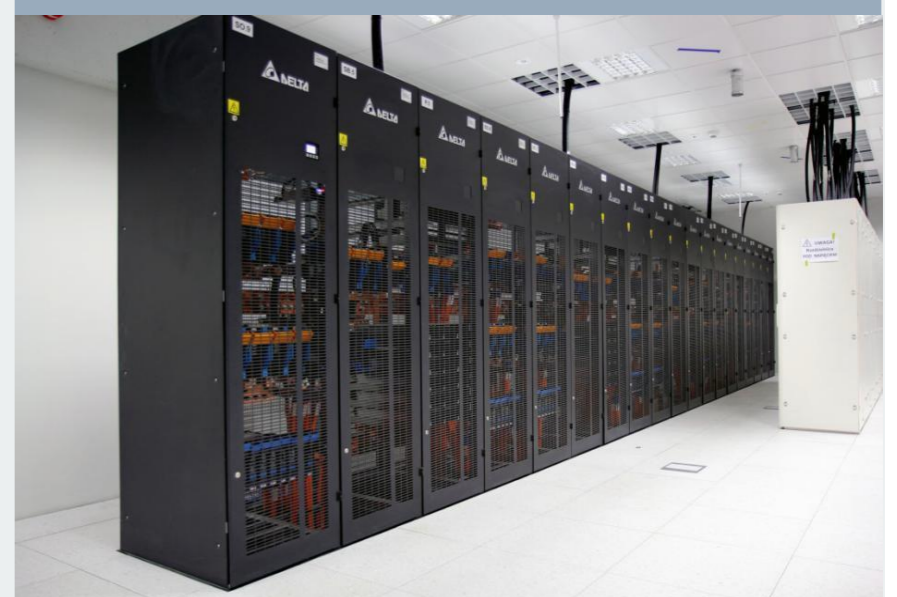
720kW Data Center application with 120 rectifiers
